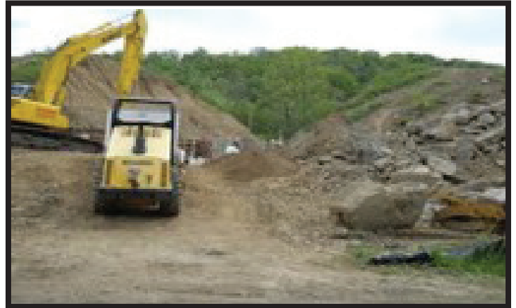
Photo: Construction of U.S. 62 tunnel in Holmes County taken last month. Photo Carolyn Lewis
